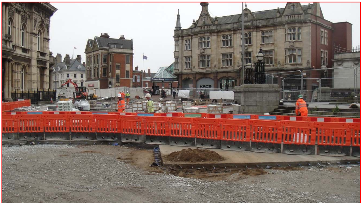
Photo Reference 19 – junction of King Edward Street and Paragon Street. Note extensive groundworks in progress at date of survey. Recommend further survey on completion of works.
